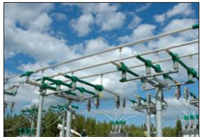
COMPLETE COVERAGE OF CRITICAL AREAS LEADS TO INCREASED POWER SYSTEM RELIABILITY
