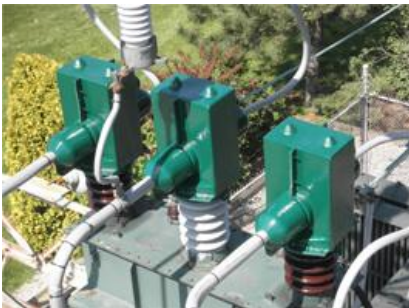
Precise Fit Cover-up for Energized Metering Equipment at Big 3 Automotive Manufacturing Facility
