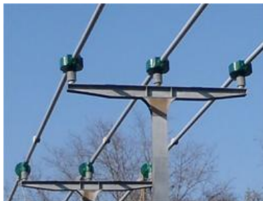
Middle Tennessee utilizes Greenjacket expansion joint covers to prevent animal and bird outages.
