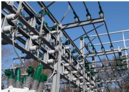
Brentwood Substation distribution bay breakers and angle bus supports protected with GreenJacket.
