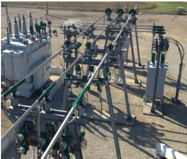
Close-up of GreenJacket installed.
